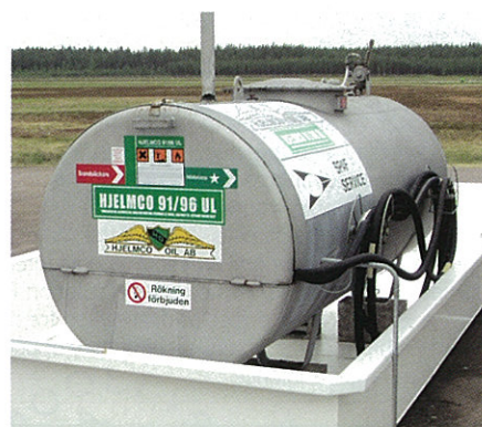
Above: Hjelmc Oil supplies unleaded avgas to more than a hundred airfields; the red dots denote where it supplies 100LL Below: one of the company's unleaded fuel bowlers in its bund
